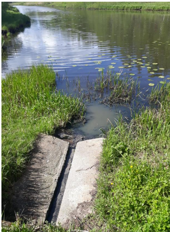
Picture 3. Before: wastewater flows into river Seda (28.05.2020.)
