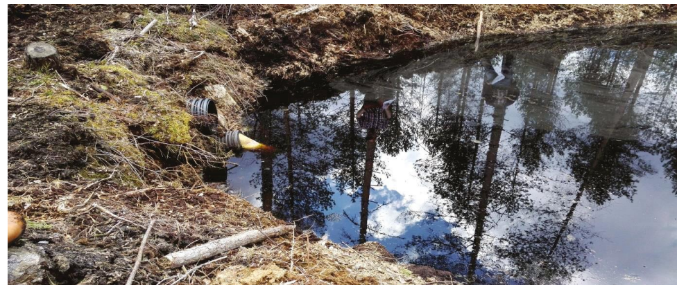
Outlet of a peak flow control structure with two pipes in a drained area located in Finland. A sedimentation pond has been constructed upstream of the peak flow control structure. Photo Leena Finér.
